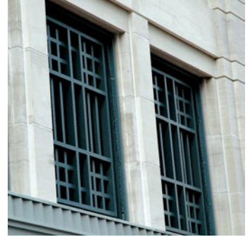
Exterior air intake grilles
