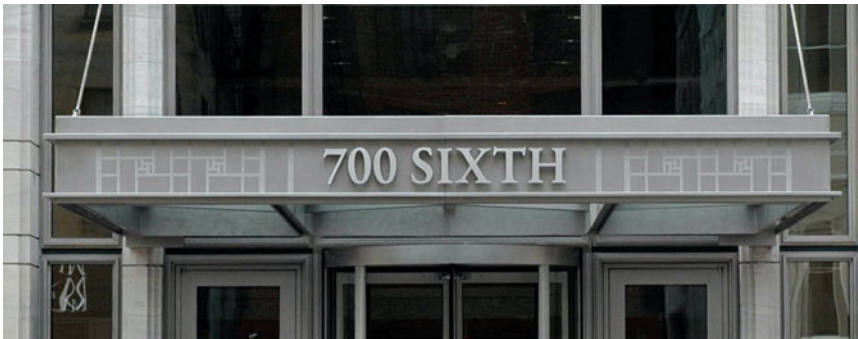
Exterior stainless steel canopy cladding
